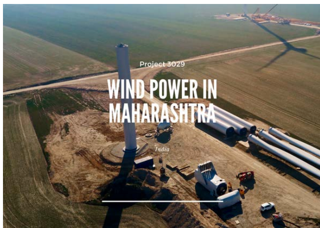
Project 3029: Wind Power in Maharashtra
